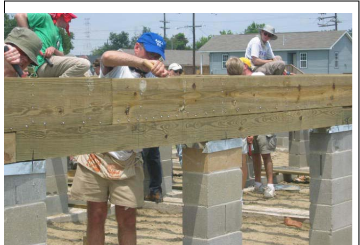
Vicky Coulter's husband Brian, working on a "floor system" at the Habitat for Humanity site in the upper ninth ward.
